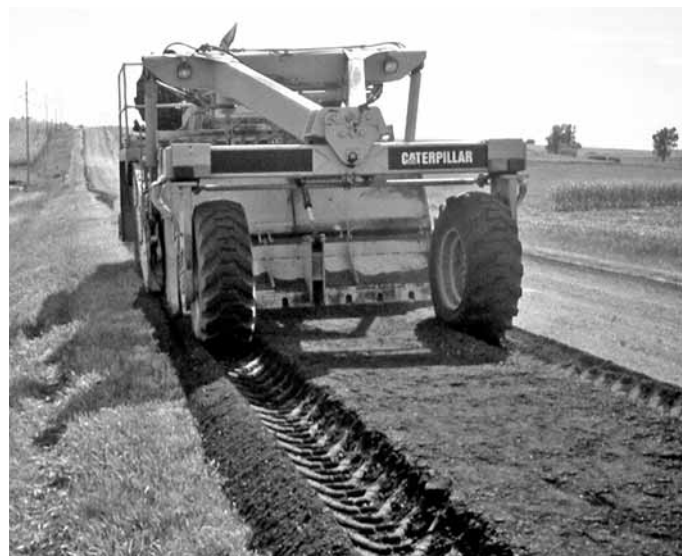
In-place recycling of asphalt surfaces is an option to consider in surface rehabilitation.
